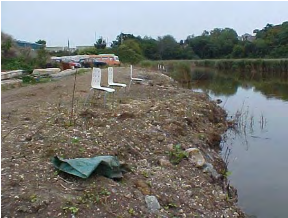
Fig 6. - Slope Filled on 6 th September 2005 where a static caravan is now situated
